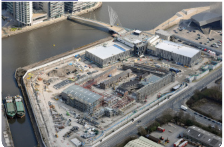
Polypipe's storm water management solutions installed at ITV's Coronation Street project, Manchester
